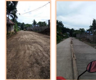
Concreting of Andres Intong St. and the Road Leading to New Calamba District Jail (2020)
